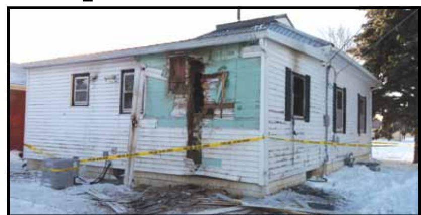
Firefighters remained on scene at this house until 11:30 p.m. checking for hot spots in the structure.
